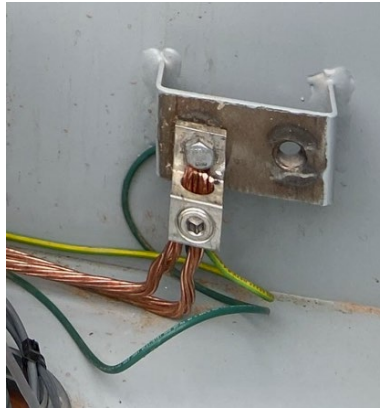
Figure 4.9—PowerDAQ ground connection
