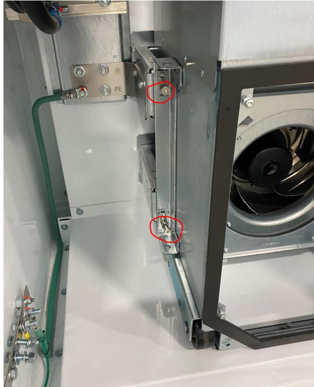
Figure 4-9: Captive Bolts at the Bottom (left side)
