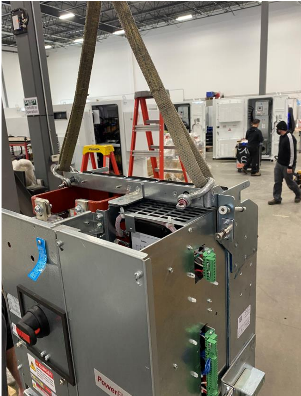
Figure 4-11: Lifting hardware attached to the lifting angle of the module.
