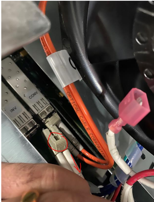
Figure 4-6: INV cable to the control pod.
