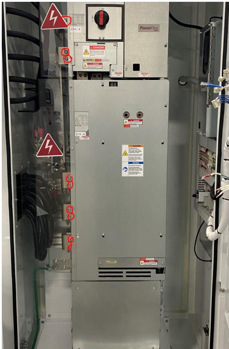
Figure 4-2: DC and AC Busbars at Drive Module
