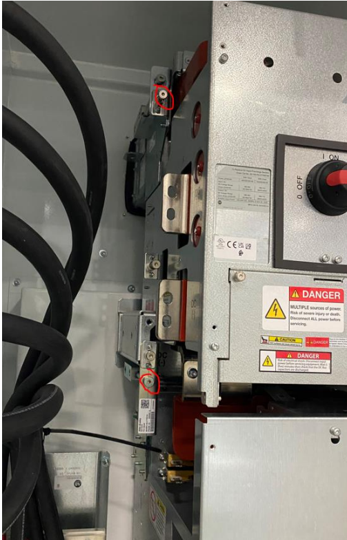
Figure 4-8: Captive Bolts at the Top (left side)
